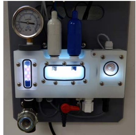
Lighted Flow Cell with CP-1 sensor, showing No Flow condition
